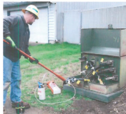
Journeyman Lineman Ryan Hardie re-energizes a pad mount transformer after working with a Novinium contractor to set up a cable rejuvenation treatment.
