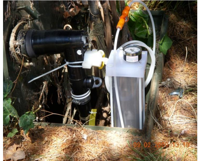
Figure 4: Injection Elbow and vacuum tank installed on a pad mount transformer.
